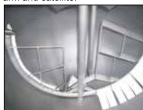
Vertical, reinforced scraper arm supported at bottom of tank..
